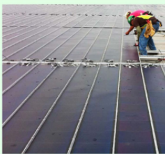
Solar Canopy system (and image credit) by Advanced Roofing
