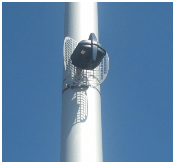
Fig. 5: Repeater (Kilde: ATKI A/S)
