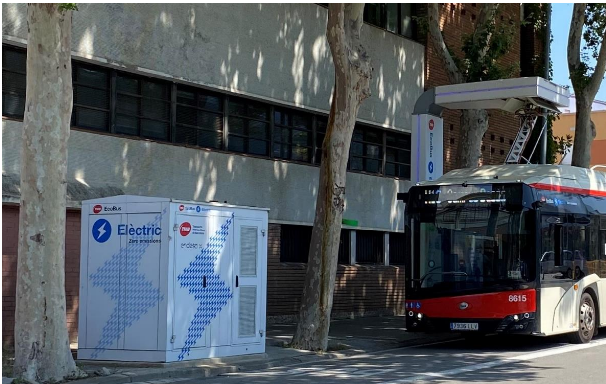
Figure 3 – Pantograph opportunity charging and infrastructure.
